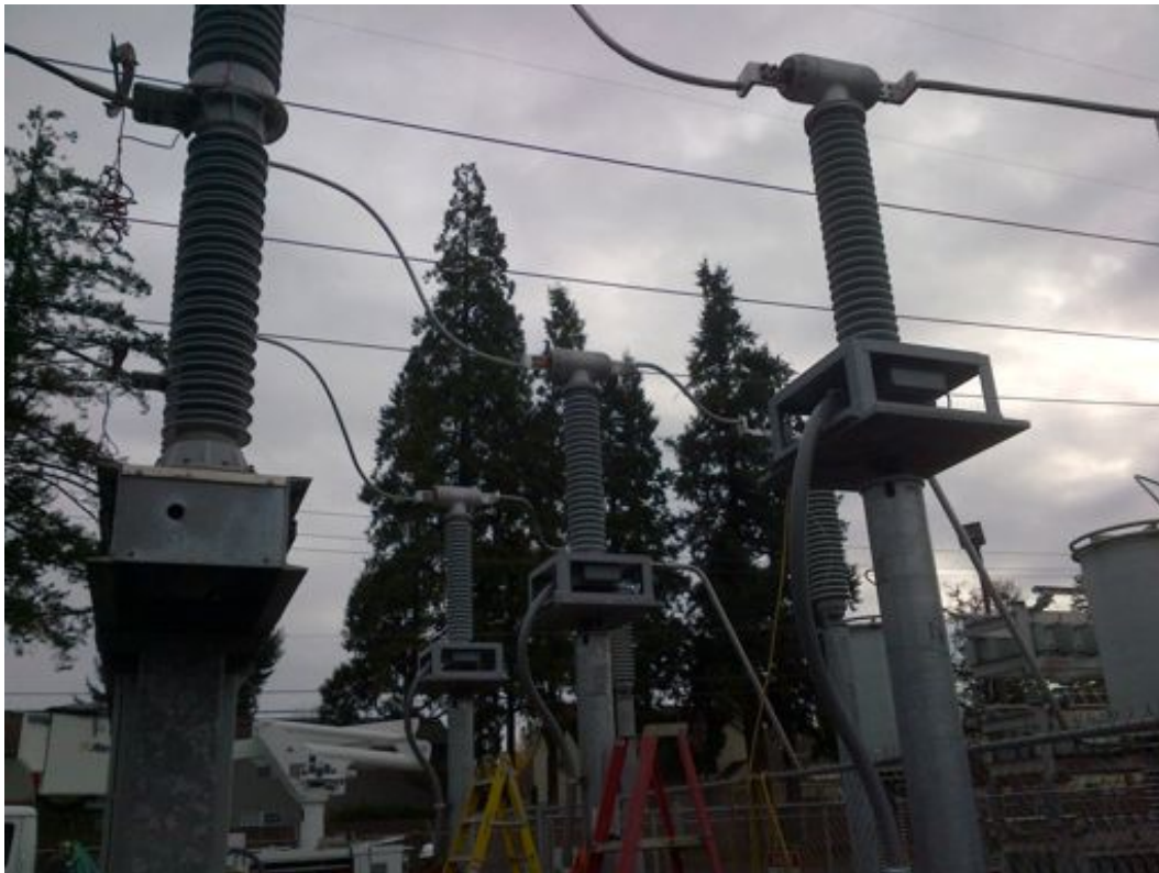
Figure 7. Electrical Phenomena Cluster (EPC), which can optically measure current, voltage, and temperature. No active electronics for E1 vulnerability instead optical cable transmits light signal to and from the control house. No conductive cabling required.
